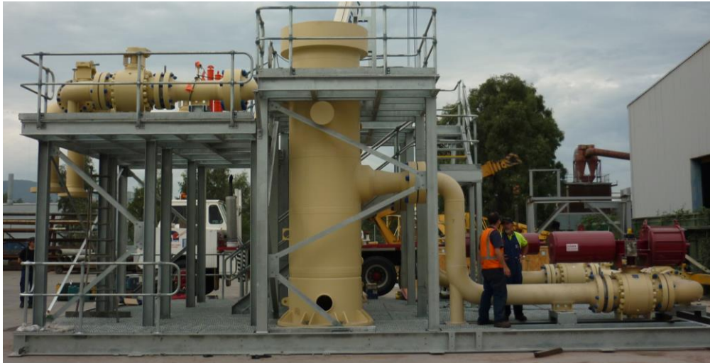
Figure 1: Typical Natural Gas Coalescing Filters in a Gas Turbine Power Station.
